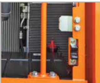
Battery cut-off switch
